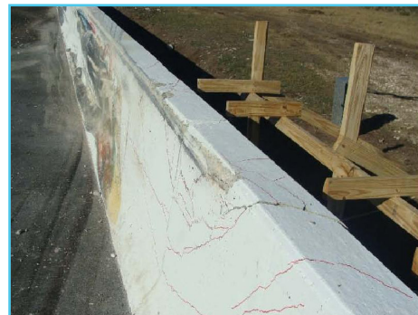
Barrier cracking as a result of tractor trailer impact during testing.
